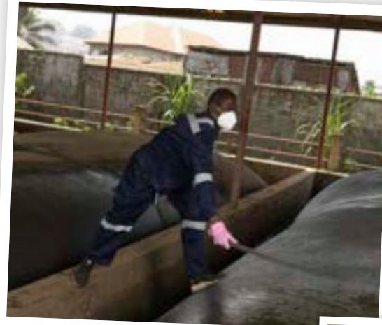
TOP: GOAL's Faecal Sludge Management (FSM) plant in Freetown, Sierra Leone.
