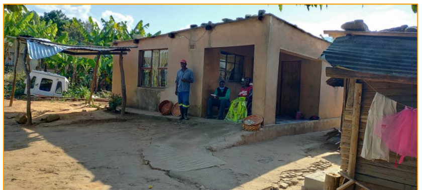
Pic 3: A repaired household - The head of household is a person living with disability, from Ward 23, Chimanimani District.
