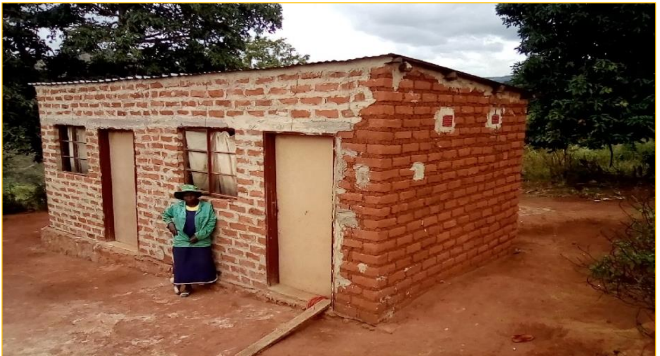
Pic 4: A house that was extensively damaged and repaired
